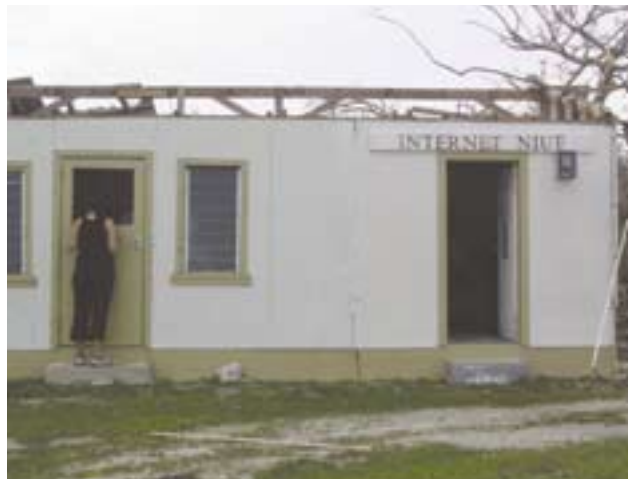
Inspecting the damage to ISU-N's Internet Cafe.
